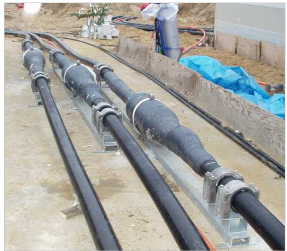
Fig. 3 : Direct buried 400 kV premolded joints
